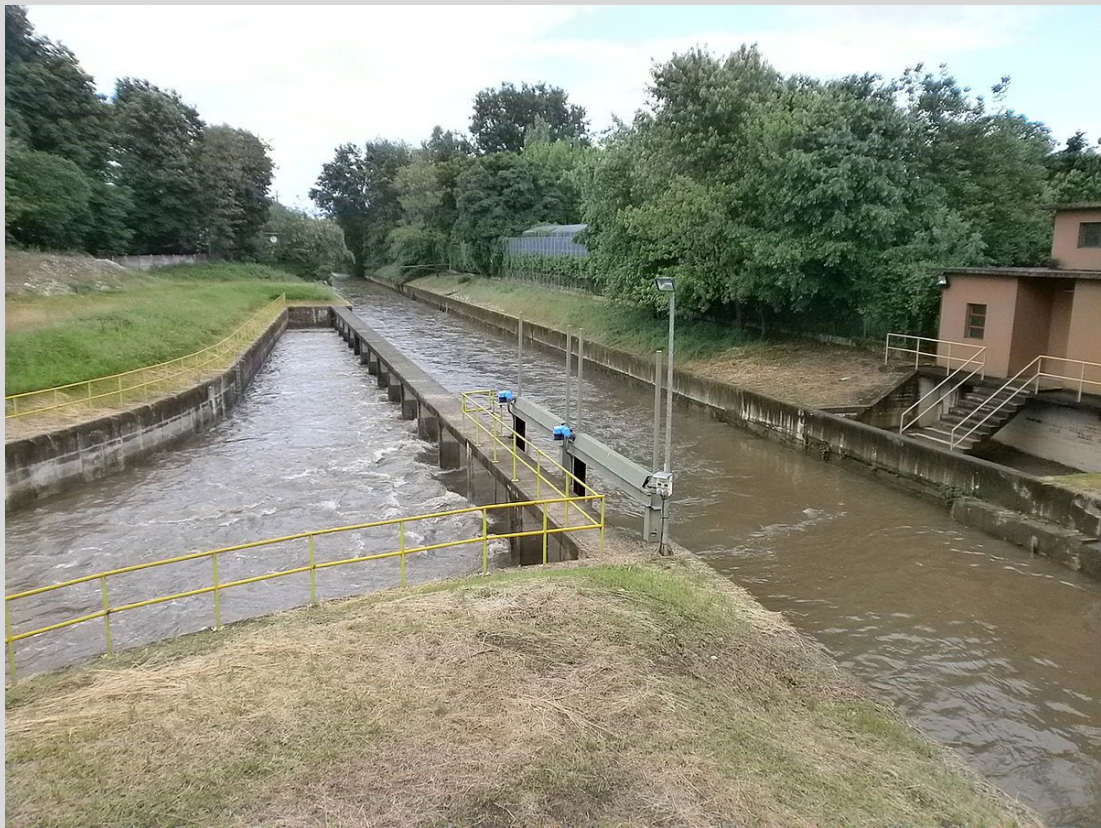
The CSNO diversion channel on the Seveso river. Image credit: Stefano Stabile, CC BY-SA 3.0, via Wikimedia Commons.
